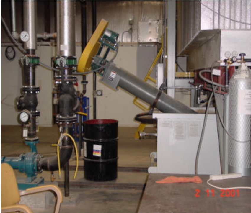
Quench Tank & Aggregate Conveyor on Demonstration Melter
