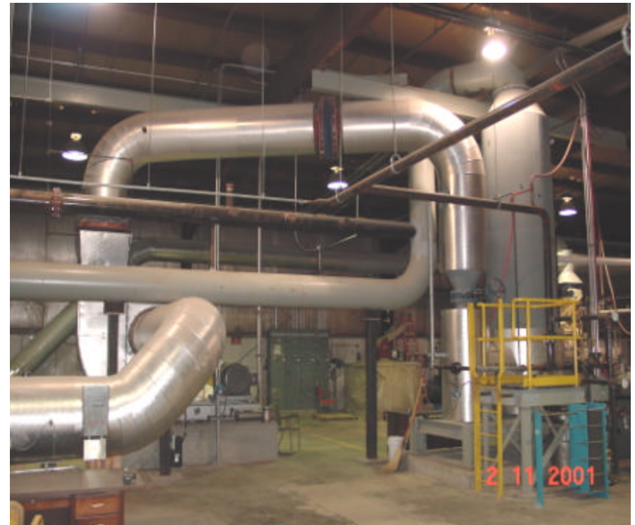
Exhaust Gas Treatment on Demonstration Melter
